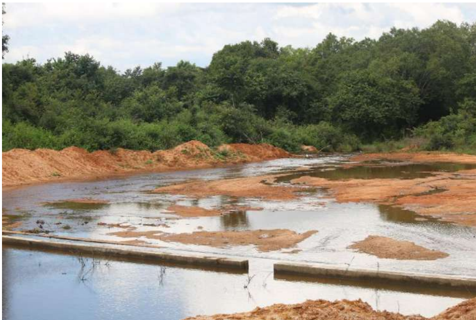
Figure 9: Repaired spillway of Thumbikulama Tank. (The spilled water runs to Bellankadawala Tank)
