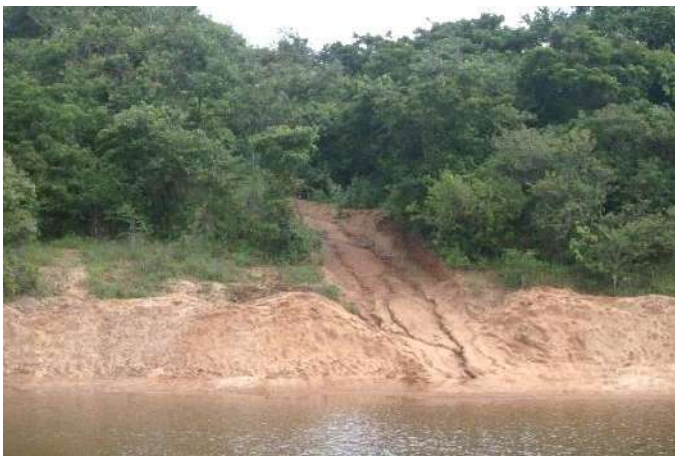
Figure 48: Soil erosion near the sluice gate of the tank
